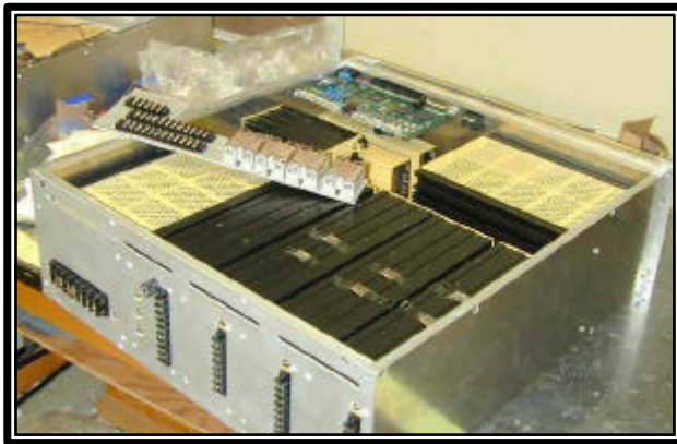
Fig. 14. Power Supply Box
